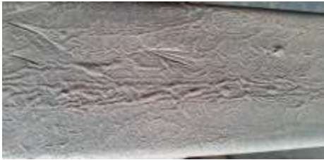
Heavily corroded structural member.
